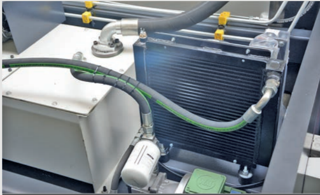
Hydraulic Oil Cooling System
